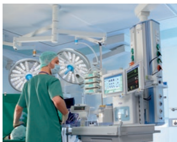
Operating theatre with a Movita ceiling supply unit
